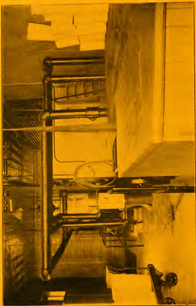
GENERAL INTERIOR VIEW OF PLANT
